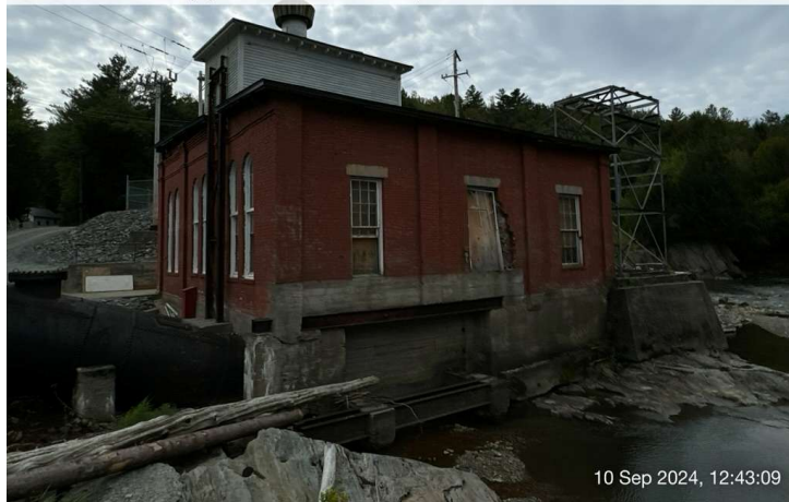
Photo 3: Tailrace (to Lamoille River) backside of the Wolcott hydropower building
