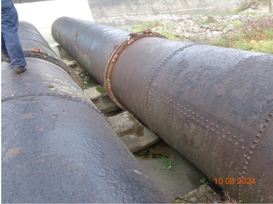
Photo 7 Right penstock at expansion joint (just upstream of surge tank); note penstock up off saddle.
