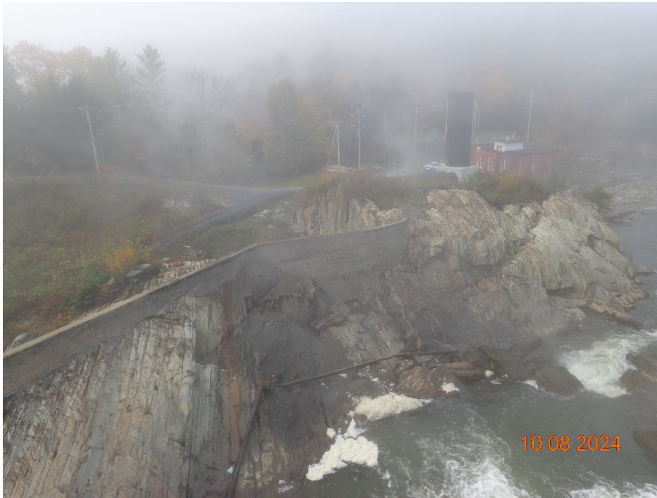
Photo 10 Looking down spillway channel from dam. Note floodwall separating the penstocks from the river.
