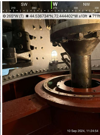
Photo 13/14: Several details view of Turbine/generator equipment
