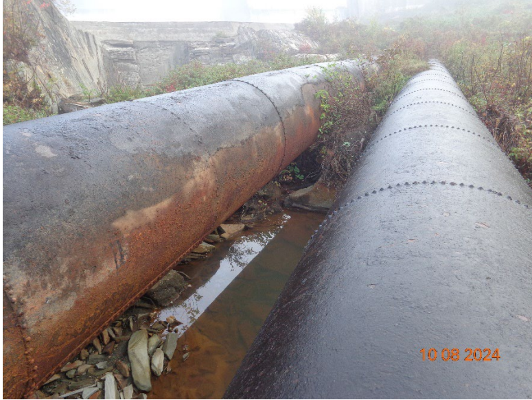
Photo 9 Right penstock looking upstream - off saddle support.
