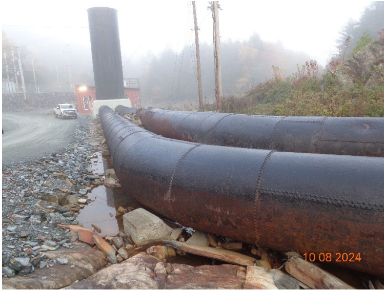
Photo 1 Looking down penstocks towards Powerhouse. Note gap between penstock and saddle support, and the remnants of material between pipes closer to surge tank
