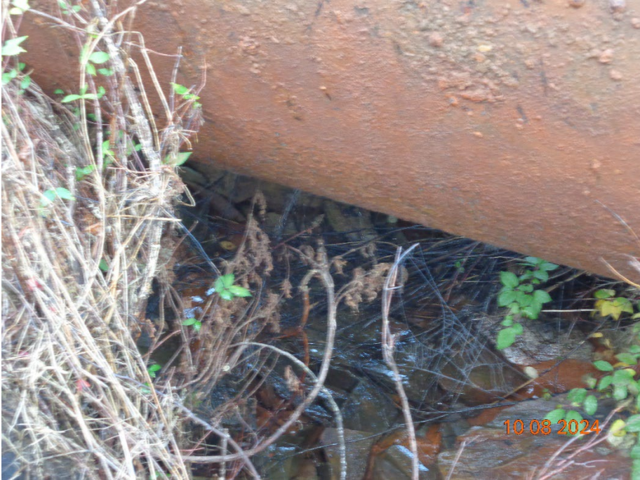
Photo 5 Leak from right penstock.
