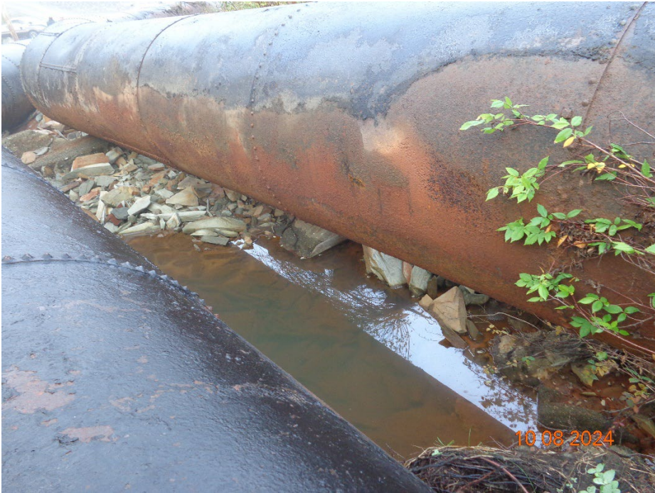
Photo 6 Right penstock undermined several feet; no longer on several saddles.
