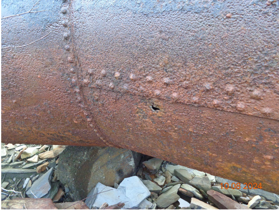
Photo 3 Hole in right penstock. Reportedly the bottom of the penstocks is the thinnest.
