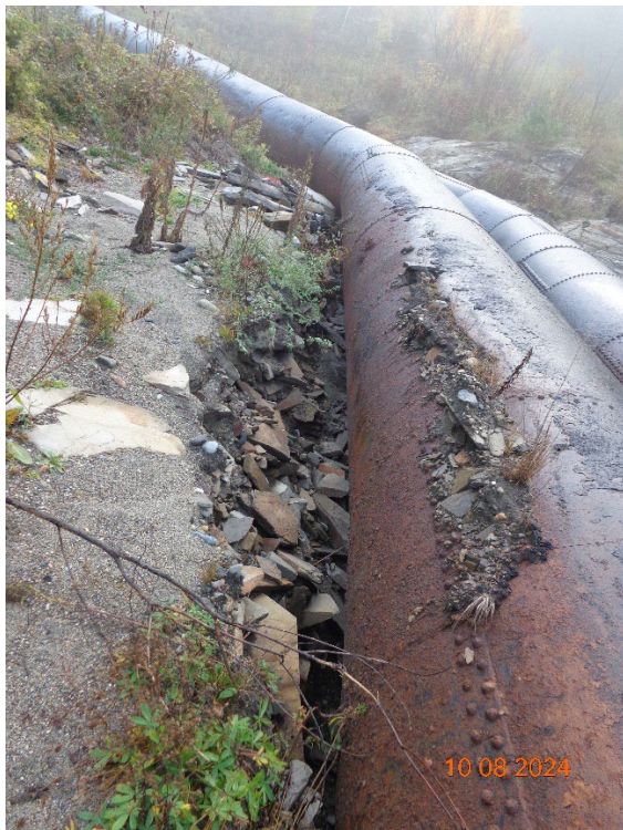
Photo 2 Looking up penstocks. Note eroded embankment on the right side and some soil on penstocks. Upper part of penstocks reportedly had a thin layer of soil (6"±) on top of pipes.
