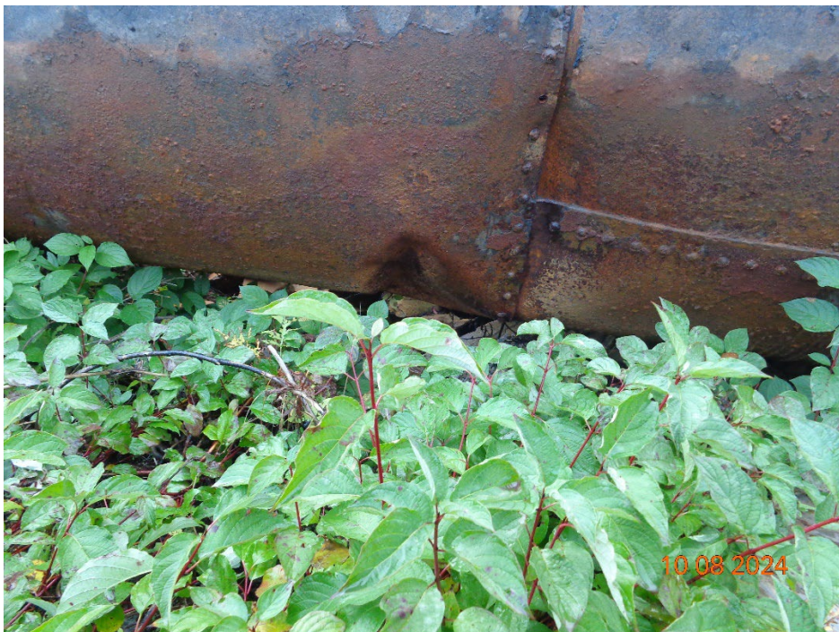
Photo 4 Dent and hole in right penstock.
